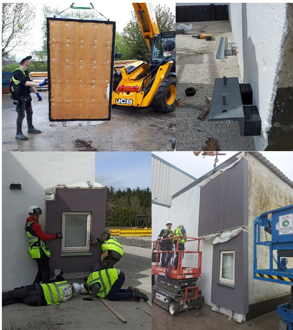
Figure 8 | Original mock-up showing - above LHS rear of panel with compressible insulation and perimeter gaskets, RHS original brackets and below - LHS first panel installation in progress, RHS wall panels installed
