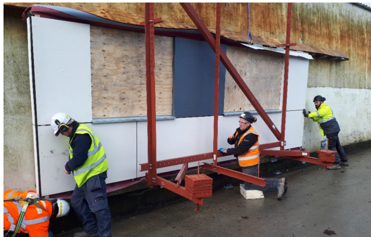
Figure 10 | Showing final mockup full scale panel installation under eaves method being tested
