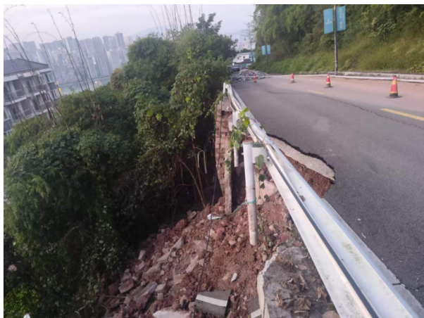
Figure 3 | Slope top roadbed collapse and pavement deformation
