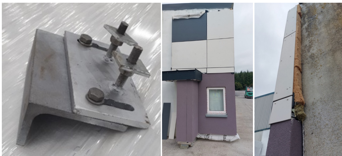
Figure 9 | Mock-up Stage 2 with LHS revised brackets allowing for minor tolerance in three planes, Centre - revised upper panels with new cement board lining and RHS – revised backing insulation
